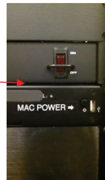
Cart and Mac Power Switches
